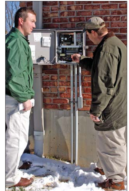
Hamilton County General Health District supervisor Chris Griffith and public health sanitarian Joe Leever inspect an electrical installation done by a Nieman crew.
